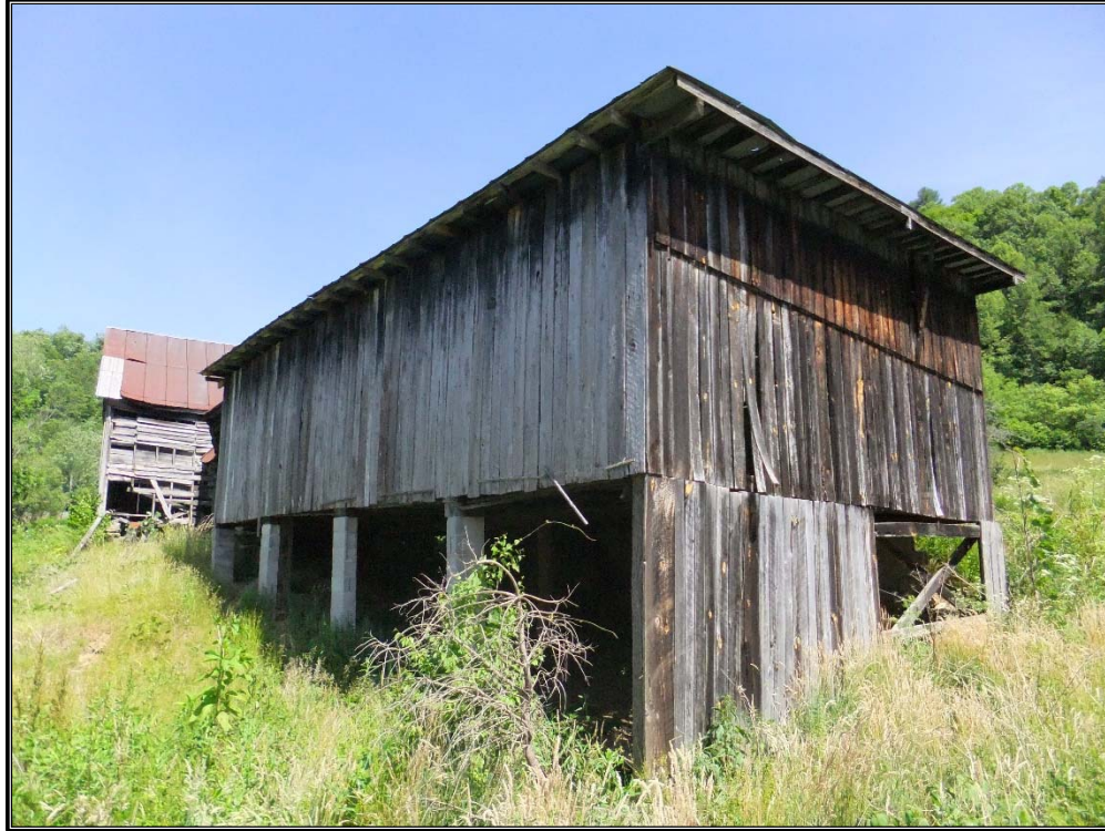
Figure 49. Rear and west elevations of the shed associated with the D.W. Tipton House (ML0129), facing east-southeast.
