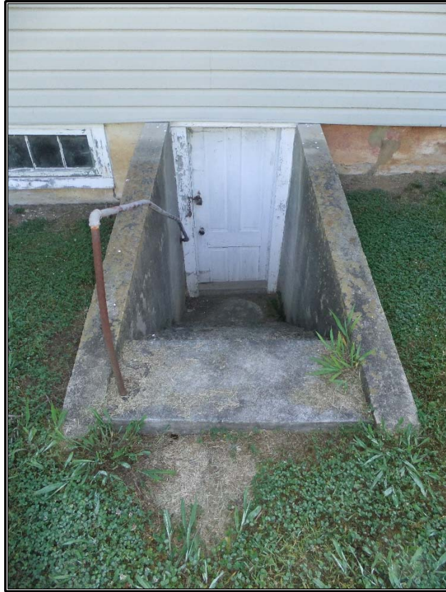
Figure 40. Basement window and wood paneled basement door of the D.W. Tipton House (ML0129), facing east-northeast.
