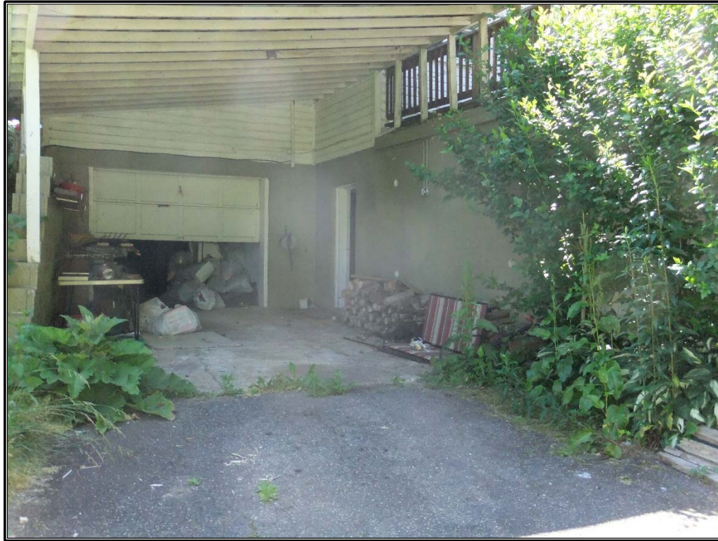
Figure 87. View of the garage of the Eston Pate House (ML0131), facing east.
