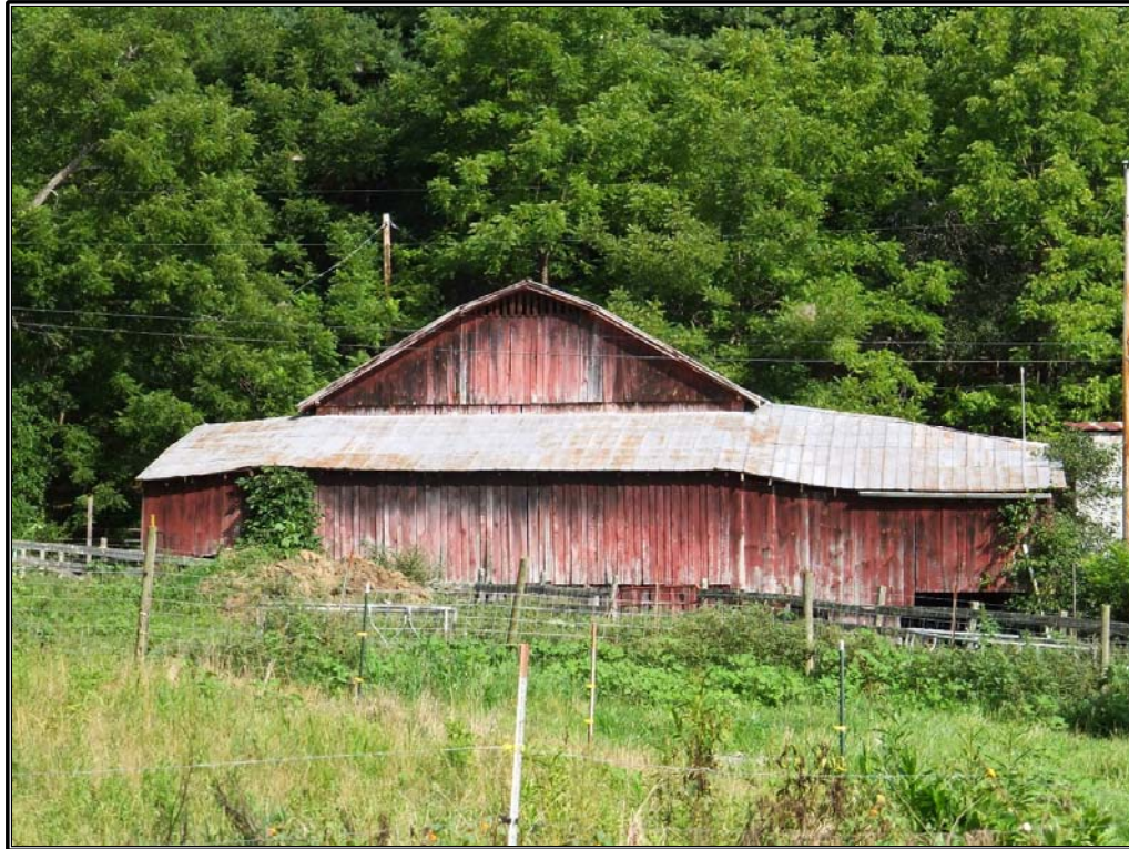
Figure 29. View of a gambrel-roof barn on NC 197 near the community of Tipton Hill in Mitchell County.
